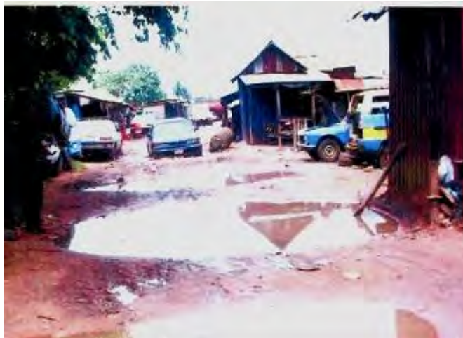
Figure 3. A typical mechanic village roadway with storm water pools.
