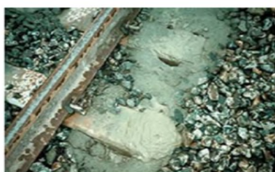
Figure 6: Ballast Mud Pumping (Burns et al., 2006)
