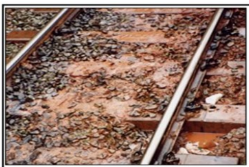
Figure 9: Subgrade mud pumping
