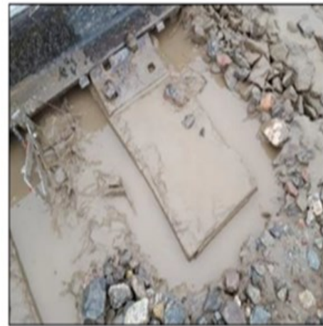
Figure 7: Ballast mud pumping with standing water (Wilk et al., 2019)
