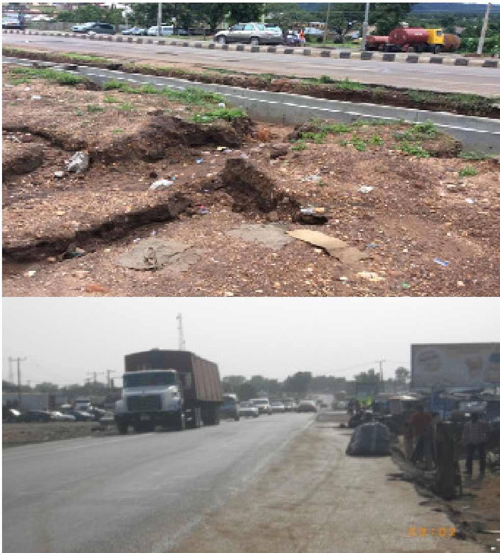
Plate 3: Road corridor with erosion due to loss of vegetation and on another side with unorganized parking space on roadside category, (mean 1.82).
