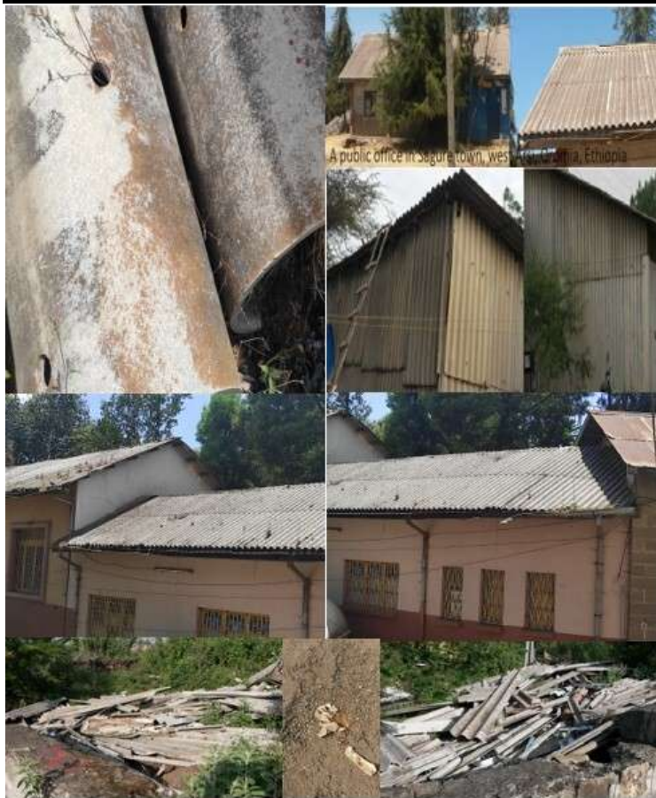
Figure 2: Concrete pipe and houses constructed using AS material in different locations of Ethiopia, and the poor management and disposal.
