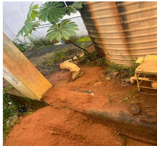
Fig 1: The Process of Extraction of Spent Sand from a Water Treatment Plant.
