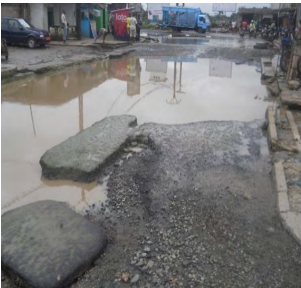
Figure4. 5 Large potholes which has widen over time during the rainy season
