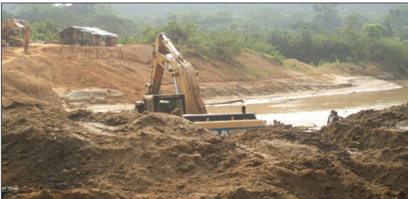
Fig 5. An excavator diverting the natural flow-path of the Ankobra River (Photo: Author)
