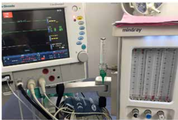
Figure 1: Anaesthesia workstation being tested after the event; connected to faulty wall gas outlet and ventilating a test lung. While supplying only medical air, note the lack of oxygen or other gas on the analyser display, subtle high flat line EtCO 2 trace and lack of capnograph reading.
