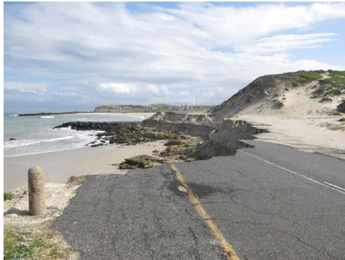
Figure 2. Photograph showing the visible coastal erosion and damage to infrastructure at the Monwabisi study area.
