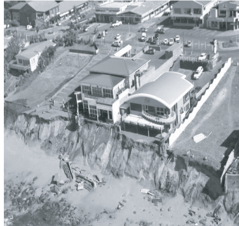
Plate 2: Damage to buildings as a result of the 2007 extreme weather event (Ballito, KZN North Coast – March 2007). (Source: Simon Bundy)
